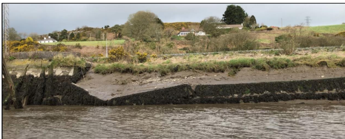
Plate 14.19 Slumping quay wall, facing north-northeast and adjacent fenders
