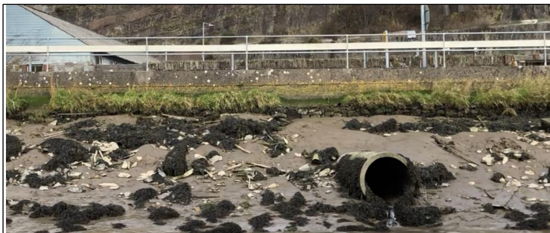
Plate 14.11 Quay wall to the west of Plate 14.10, showing outfall and denuded wall, facing north
