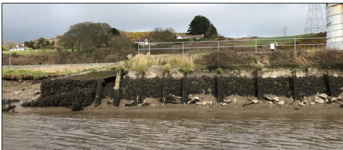
Plate 14.18 Timber fenders along quay wall and area of adjacent collapse, facing north-northeast
